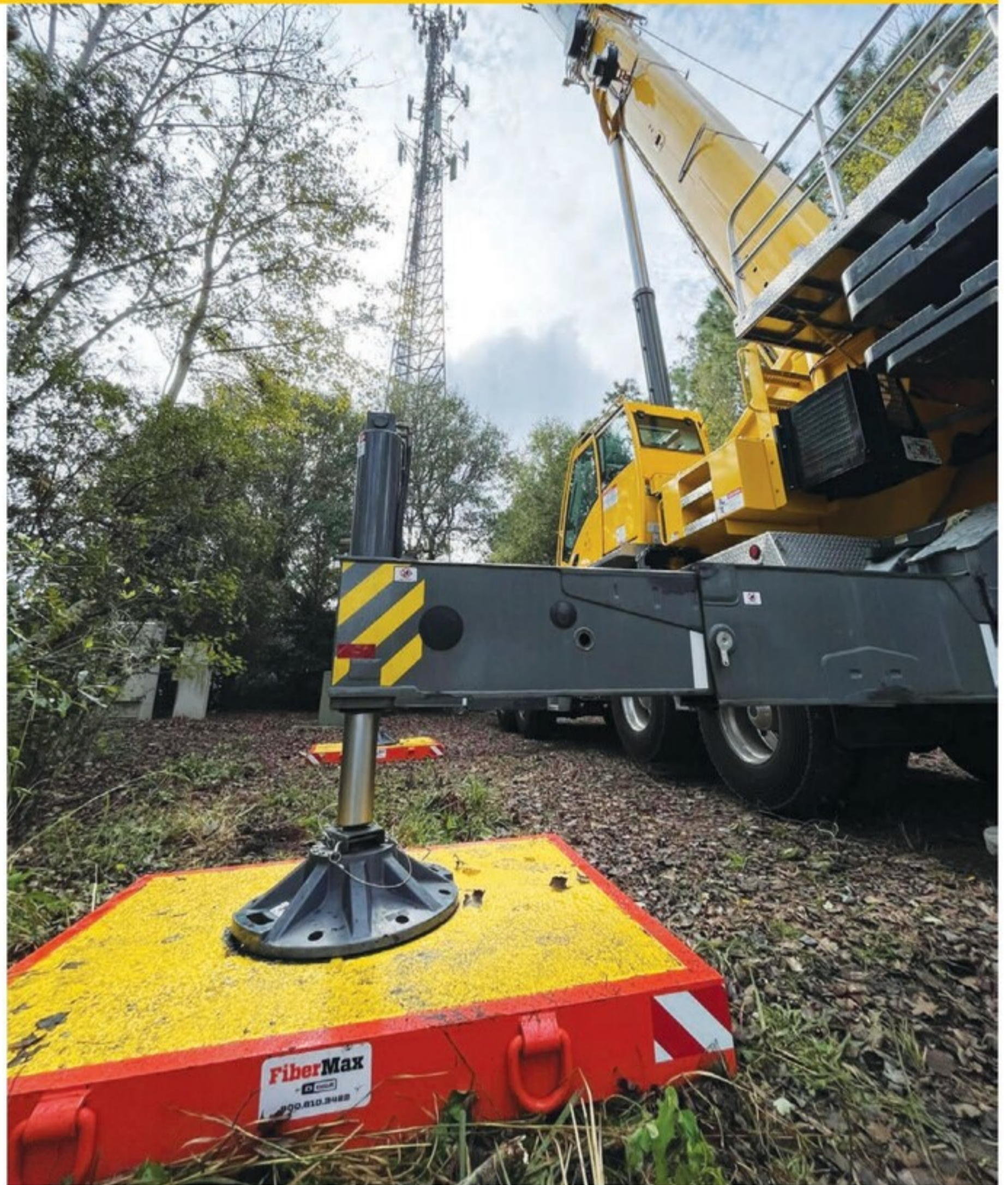
▲ Stiffness is required to spread the load, and the combination of both strength and stiffness is required to prevent the crane from going out of level.
